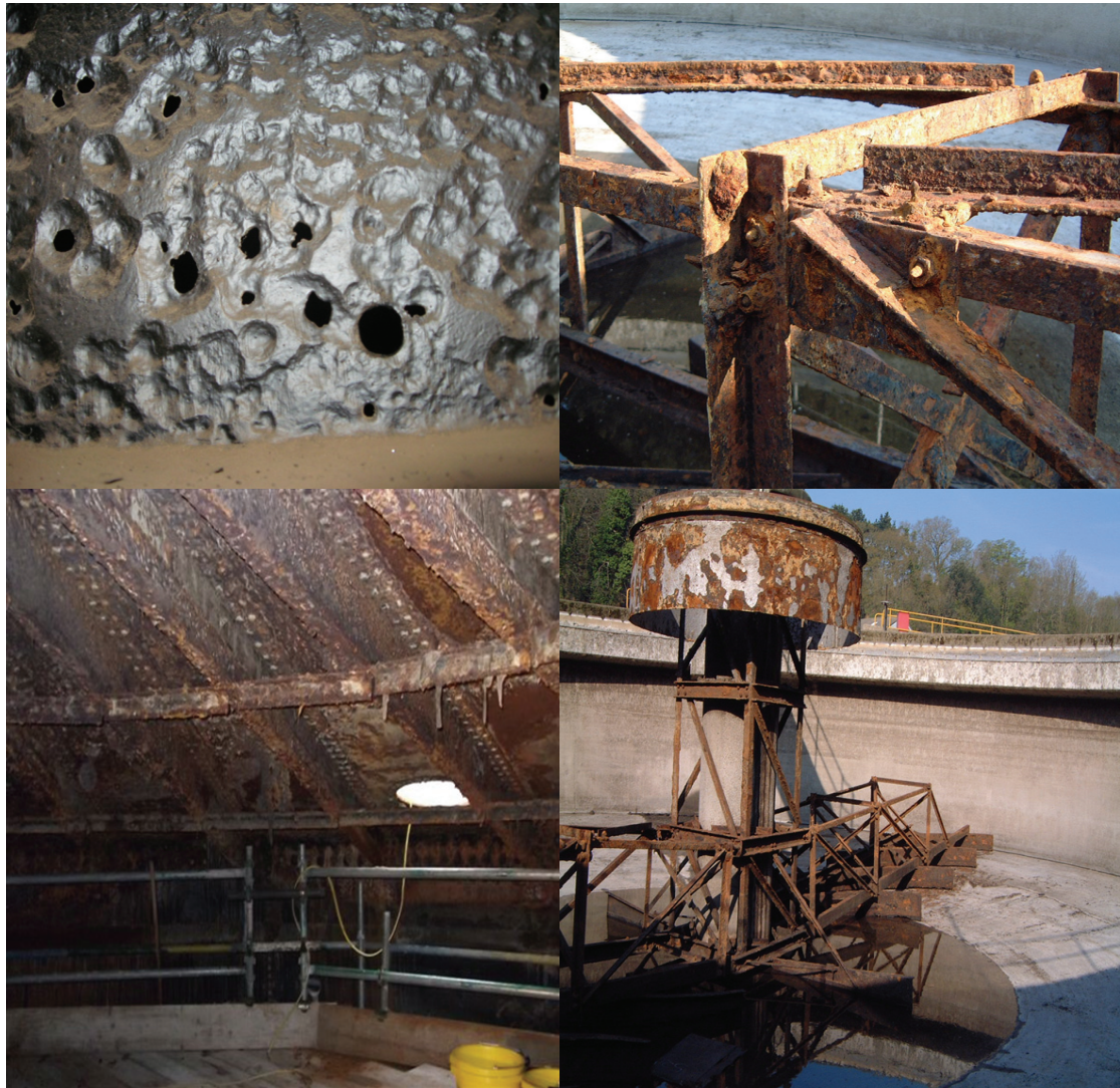
FIGURE 72 – AGEING SEWAGE TREATMENT WORKS
